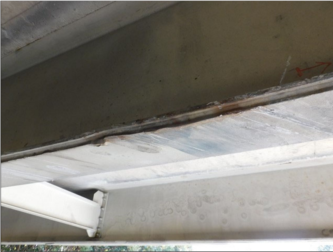
Span 2 Beam 9: ALONG BOTTOM FLANGE AT MID SPAN, AREA OF IMPACT DAMAGE [6 FOOT LONG] WITH DEFLECTION [UP TO 1/2 INCH].
