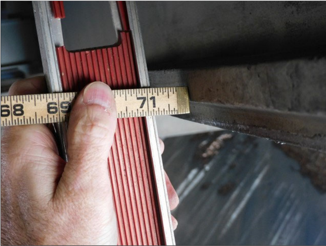
Span 2 Beam 8: LOCATED 18.5 FEET FROM INTERIOR BENT 1 - ALONG MIDSPAN OF BOTTOM FLANGE AND COVER PLATE, AREAS OF IMPACT DAMAGE [4 FOOT X UP TO 1 INCH DEFLECTION]
