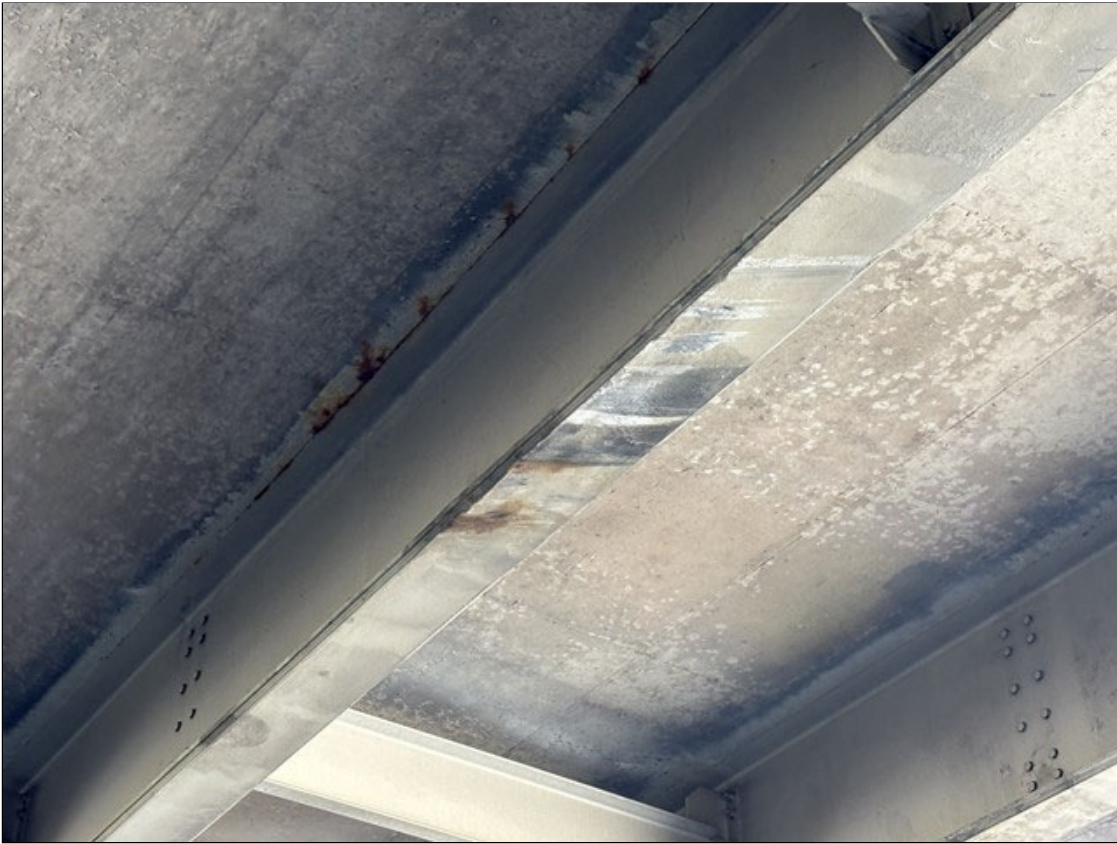
Span 2 Beam 8: (2) AREAS OF IMPACT DAMAGE UP TO 4 FOOT LONG WITH UP TO 1 INCH DEFLECTION IN LEFT EDGE OF BOTTOM FLANGE AND COVER PLATE, AT 17 FOOT AND 18 1/2 FOOT FROM BENT 1
